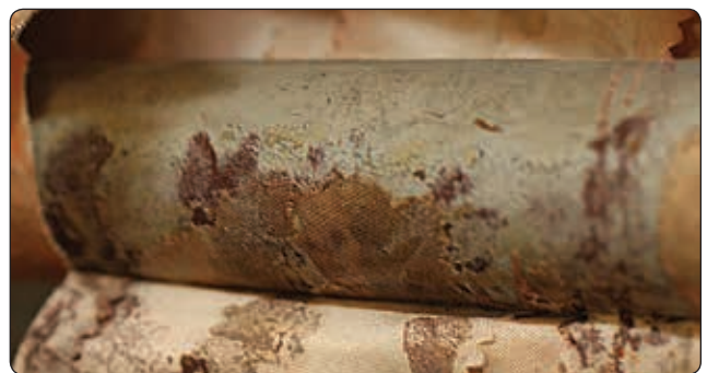
Figure 8-27. Rust on structural components.
