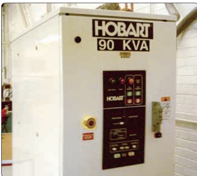
Figure 1-28. A stationary electrical power unit.
