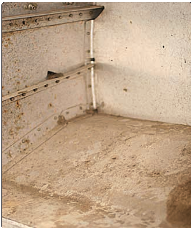
Figure 8-4. Direct chemical attack in a battery compartment.
